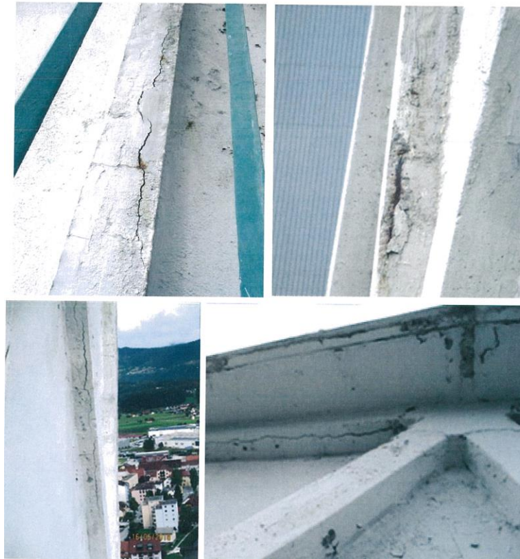
Figure 2: On diagonal in horizontal elements there are cracks, falling of concrete cover
