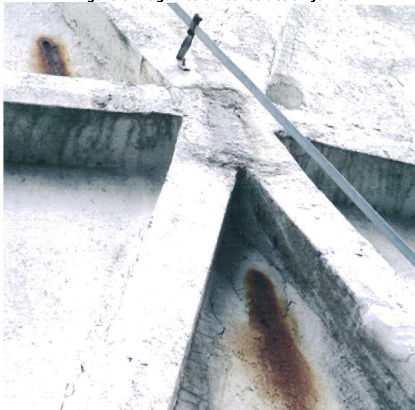
Figure 7: On the RC filling sabs corrosion stains are visible due to highly corroded reinforcement
