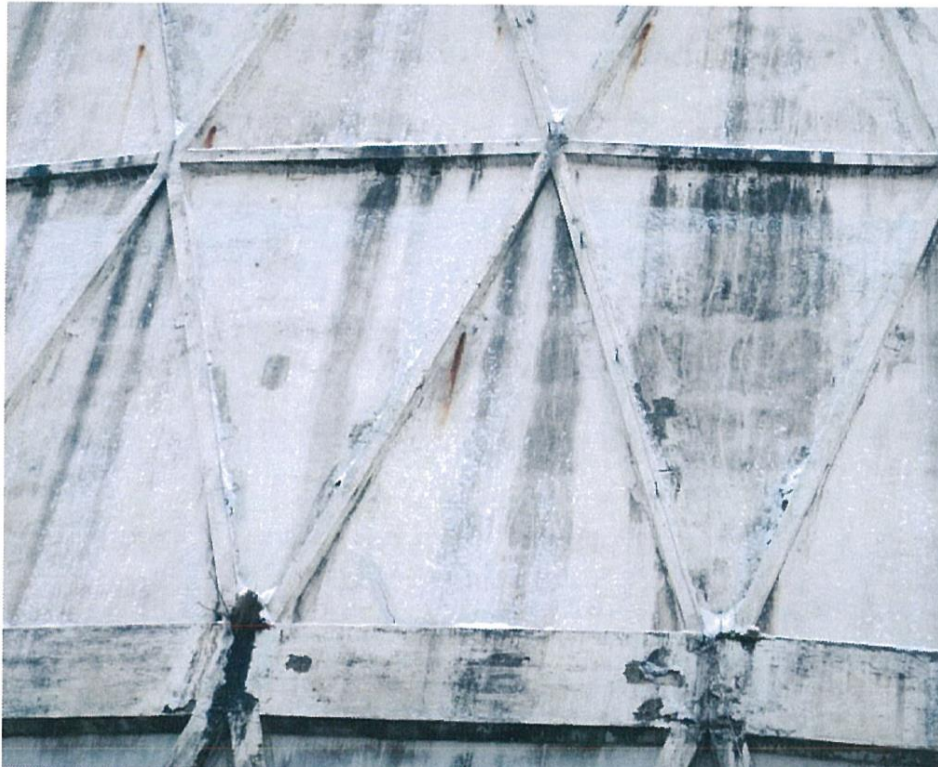
Figure 4: Damages on the RC filling slabs together with dirt
