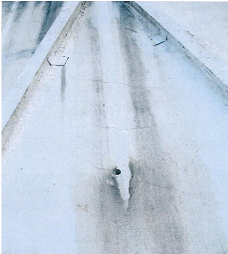
Figure 5: Cracks in the RC slab elements
