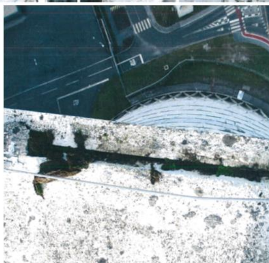
Figure 9: Brace ring damages
