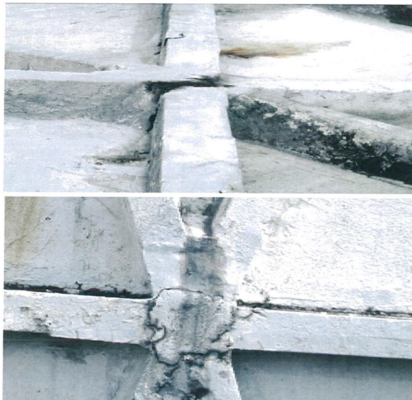
Figure 3: Damages at joints
